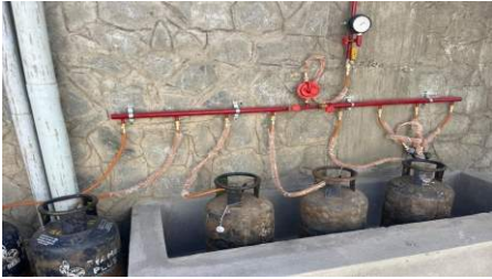
Gas Line maniFold
